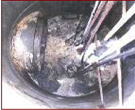
Before addition of FOG 2000 with BioS 3112: 90% of lift station water surface was covered with a grease cap. The darkened, crusty areas on top of the grease indicates thick and aged grease in the lift station
